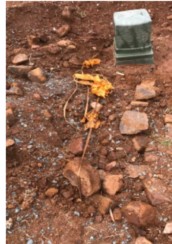
Figure 3: Signaltape Prevented Damage #1
