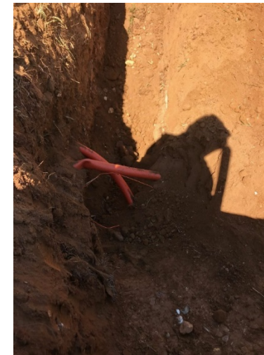
Figure 2: No Signaltape installed above Ting Conduit
