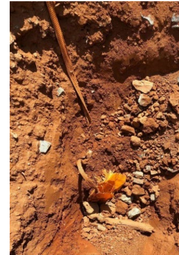
Figure 4: Signaltape Prevented Damage #2
